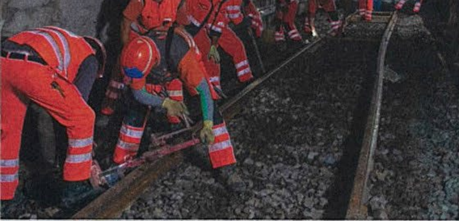
Track workers place a hand-pumped jack to lift a new rail over ballast and into place inside a Swiss tunnel.
